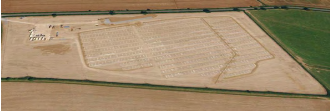
Total site strip (Blisworth site) removing all vegetation on Applicant's industrial solar site at initial construction phase
